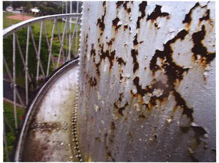
Tank shell coating and cat walk.
