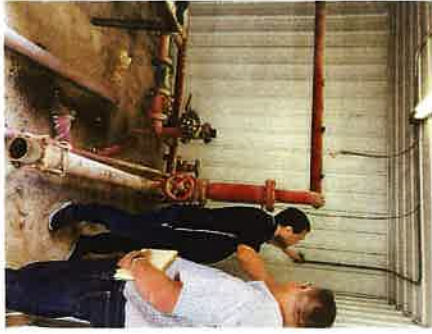
EXISTING PROCESS PIPING
