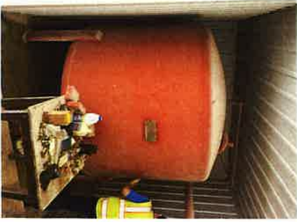
EXISTING SAND FILTER
