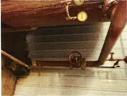
EXISTING PROCESS PIPE & VALVE
