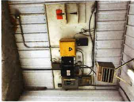
EXISTING ELECTRICAL EQUIPMENT
